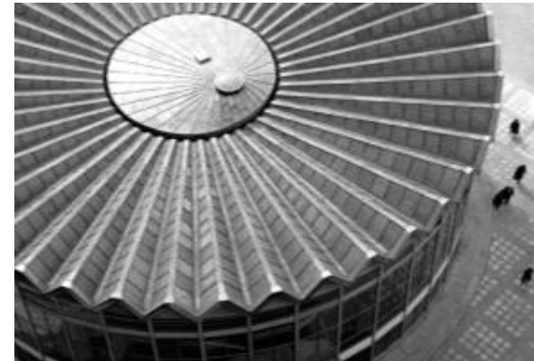
at present – poor technical condition, BUT: Rotunda considered an icon of the city
